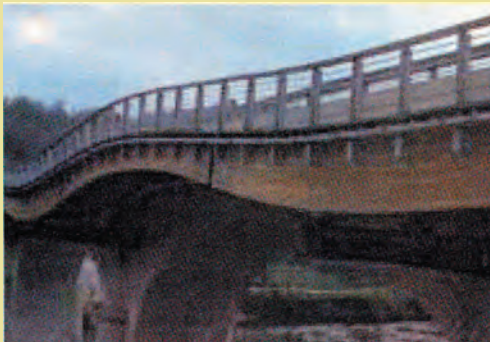
Wooden footbridge for pedestrians and cyclists fixed by means of cantilevering supports along the side of the Pont des Eyzies over the River Vézère
