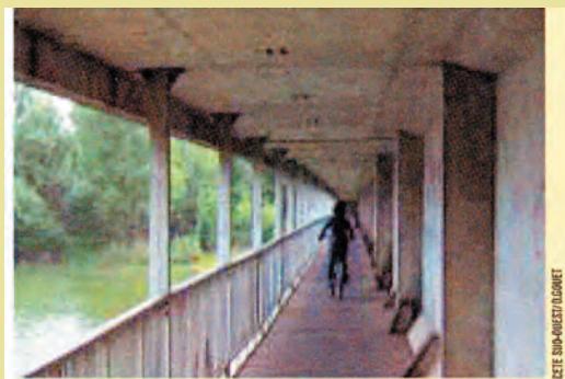
Covered crossing built into an existing motorway bridge, running below the road, ensures the continuity of the Lac de Bordeaux greenway; a heavily-congested ring road with dual-lane traffic in each direction runs across the bridge itself
