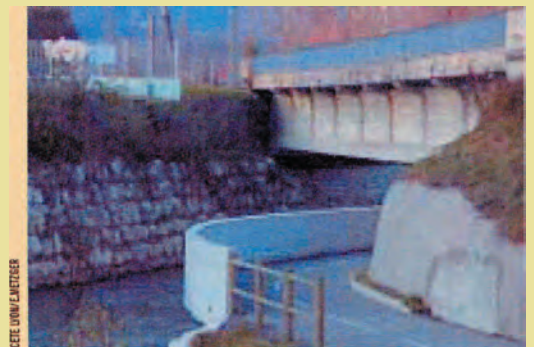
Chambéry to Lake Bourget route passing under an existing structure by means of corbelling; a line down the middle divides the path into two, with a lane for traffic in each direction, thus ensuring safety for cyclists
